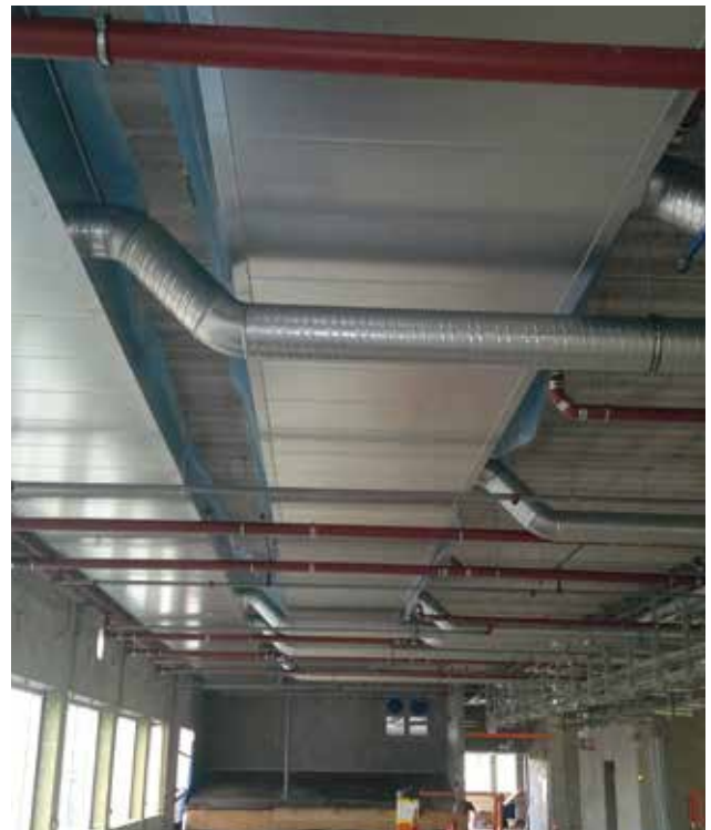
Noise-dampening for ventilation ducts and shafts. New Karolinska Solna, hospital in Solna, Sweden.
